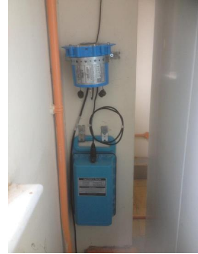
Data Logger & Battery pack
